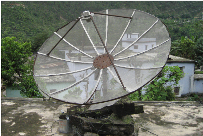
a satellite dish on the roof
